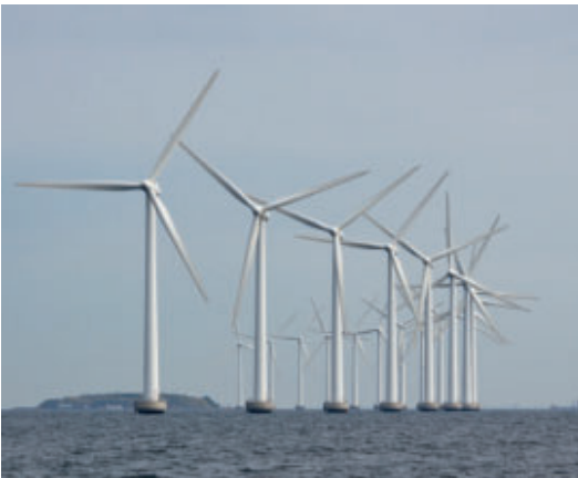
5 Danish offshore wind farm
